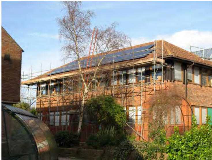
Solar panels at Chiltern District Council offices
